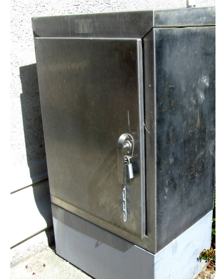
Above: The smart irrigation control box next to Wellman.
